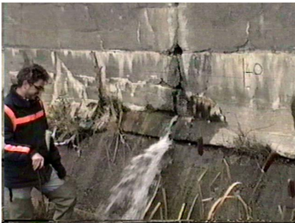
Fuites Seepage (Leaks)
