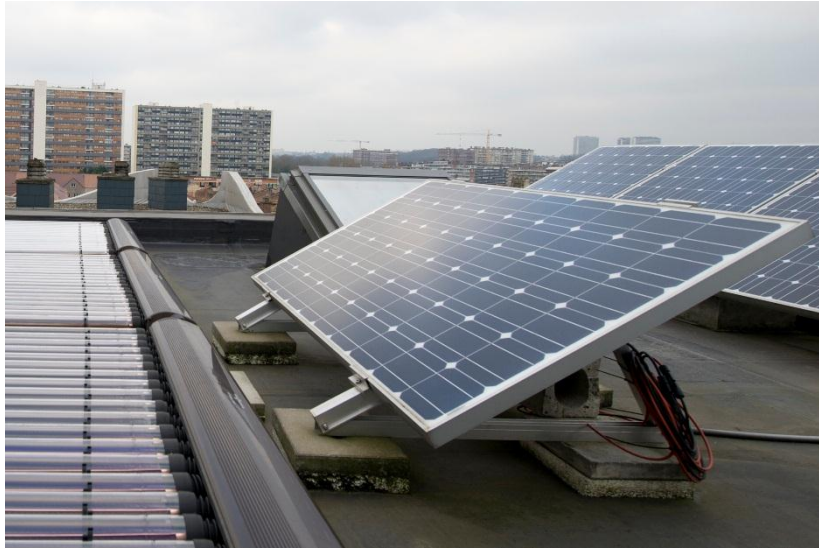
Figure 29: installation photovoltaïque inclinée
