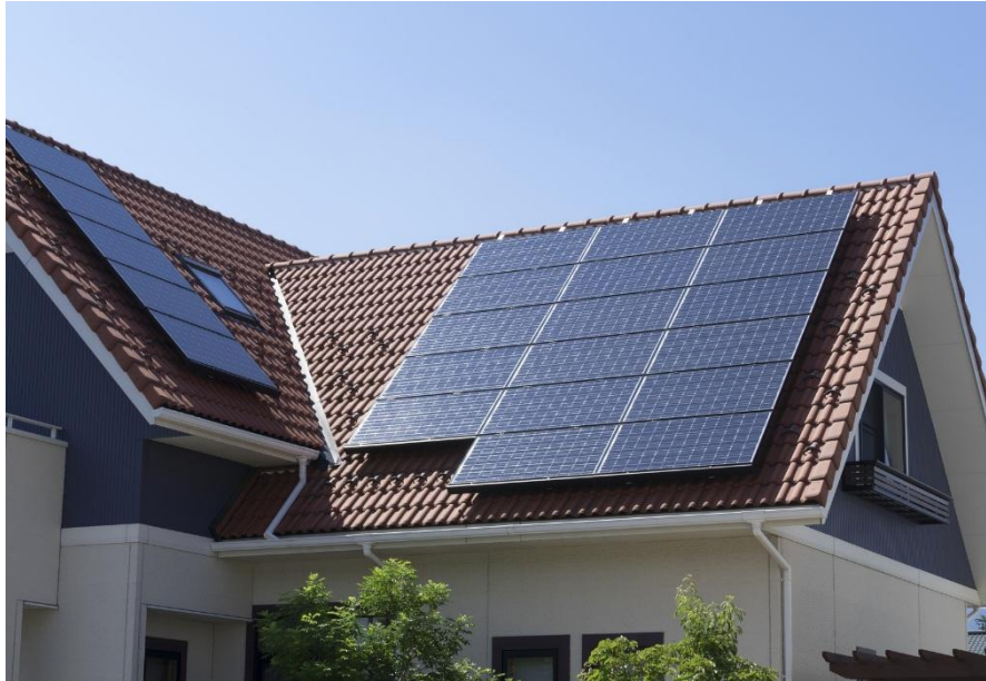
Figure 28: installation photovoltaïques non-incliné.
